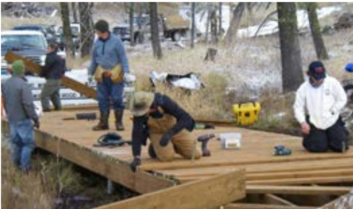
Volunteers and professional carpenters helped us build the Boulder Creek Boardwalk in Donnelly in a matter of days.
