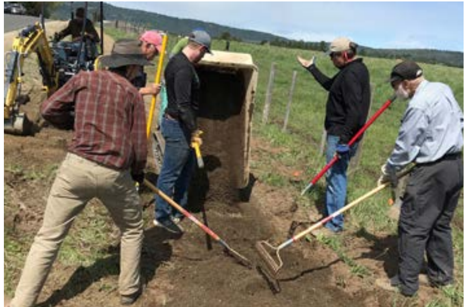
Volunteers pull wet road mix out of the Mud Buggy and spread it 4-6" deep across the trail. Then, Payette Environmental rolled the trail with an Ingersoll-Rand compactor, and the Southern Idaho Timber Protective Association watered it to finish off the project.
