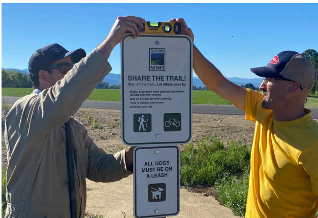
Wes Keller, left, and Tyler Busby install trail signs on the Heinrich Demo Trail.
